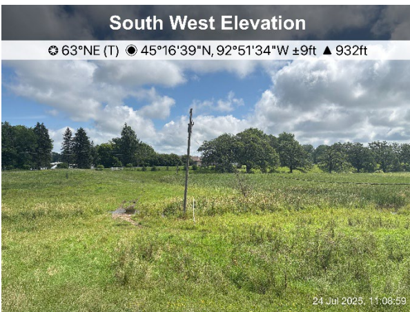
Photo 21: North end/former farmstead area facing northeast, overhead powerline pole with transformer, no signs of leakage
