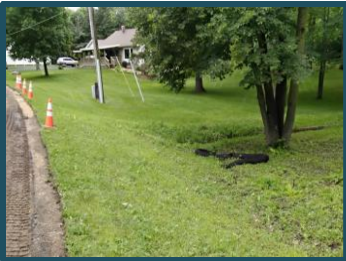
Photo from June 27, 2025 report requesting additional biolog ditch checks and stakes
