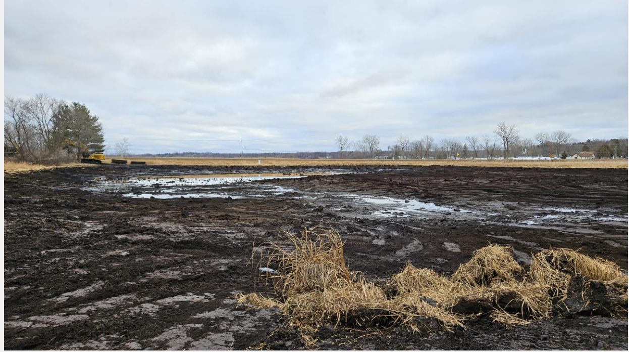
WJD6 Wetland Project Area. Excavation completed. Salvaged native sedge mats in foreground.
