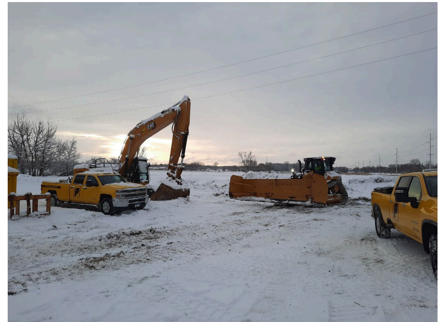
Site prep continues at the project site in order to drive frost.
