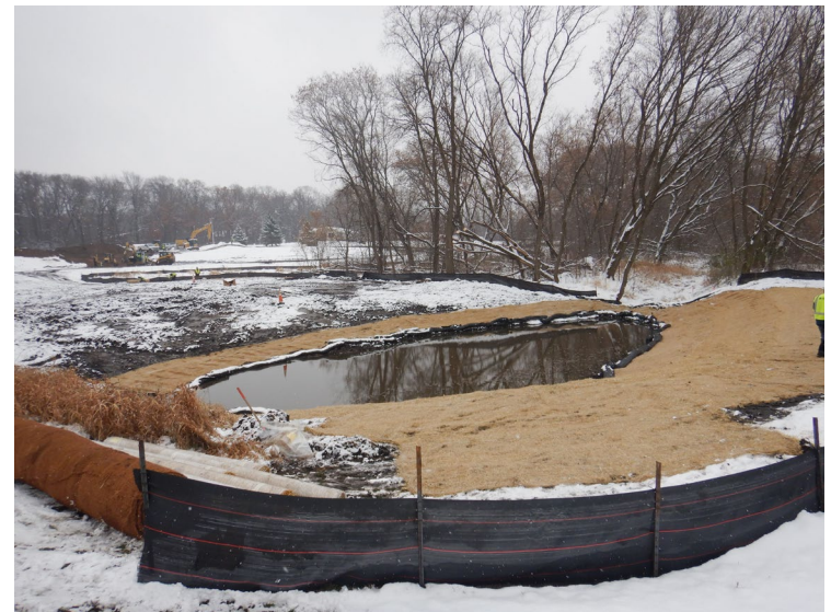
Ditch intake pool.
