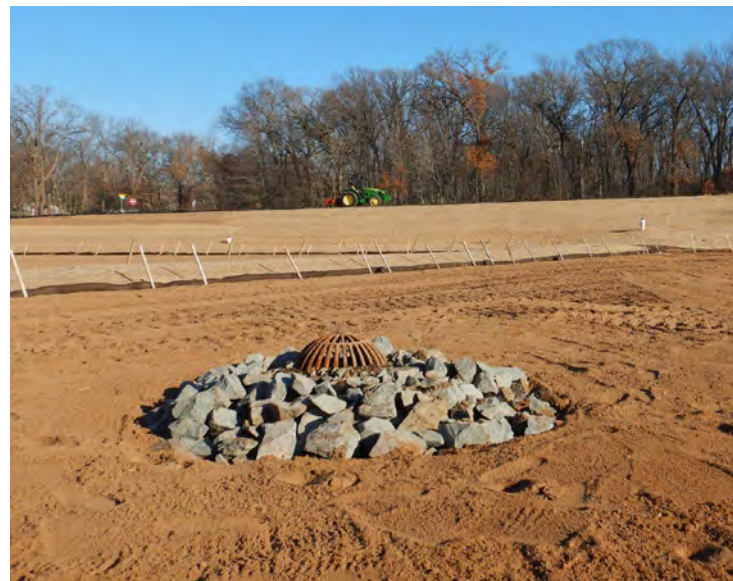
Sand filter inlet structure.
