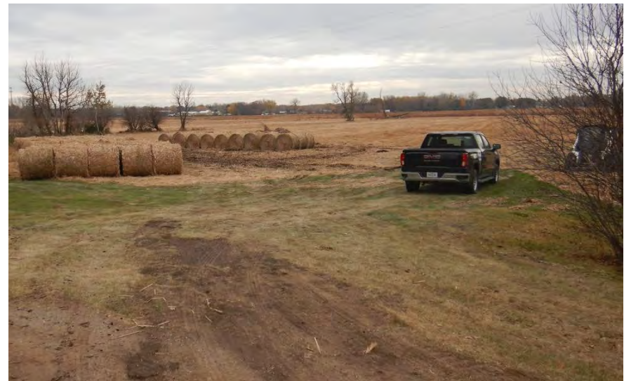
Site prep – vegetation cleared to help drive frost. All bails have been removed.
